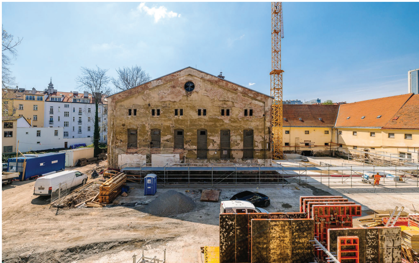
Figure 18 Restoration of the brewery historic building under way in 2023, the picture shows the future square, source: nuselskypivovar.cz
